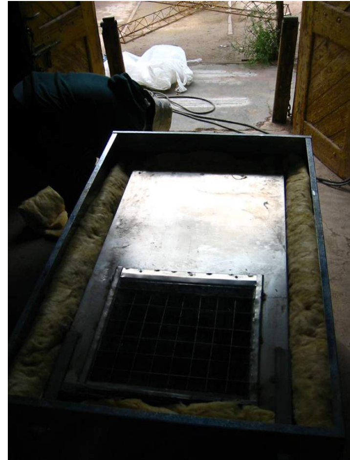
After all parts are finished the oven can be insulated with mineral or rock wool. The spacing between inner and outer wall is 10 cm. All in all 8 m 2 of mineral wool is needed.
